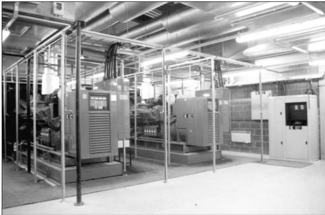
Twin 800 DFHD sets (1000 kVA) with QST30 G4 engines, PCC control and DMC autosync cubicle in a typical installation.
