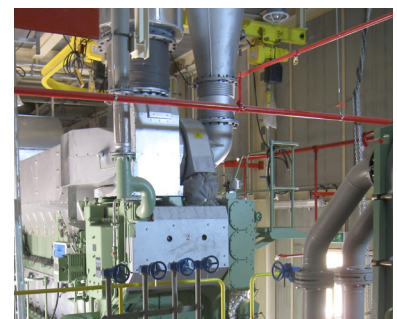
Inside view of Enclosure(Pre-fabricated type)
