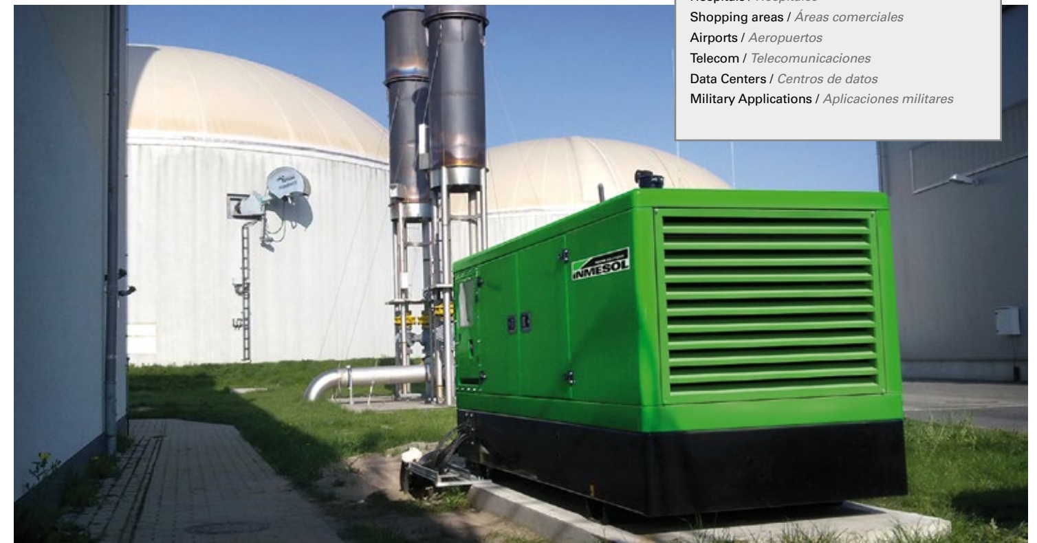
Industrial generator set in a business in Belgium
