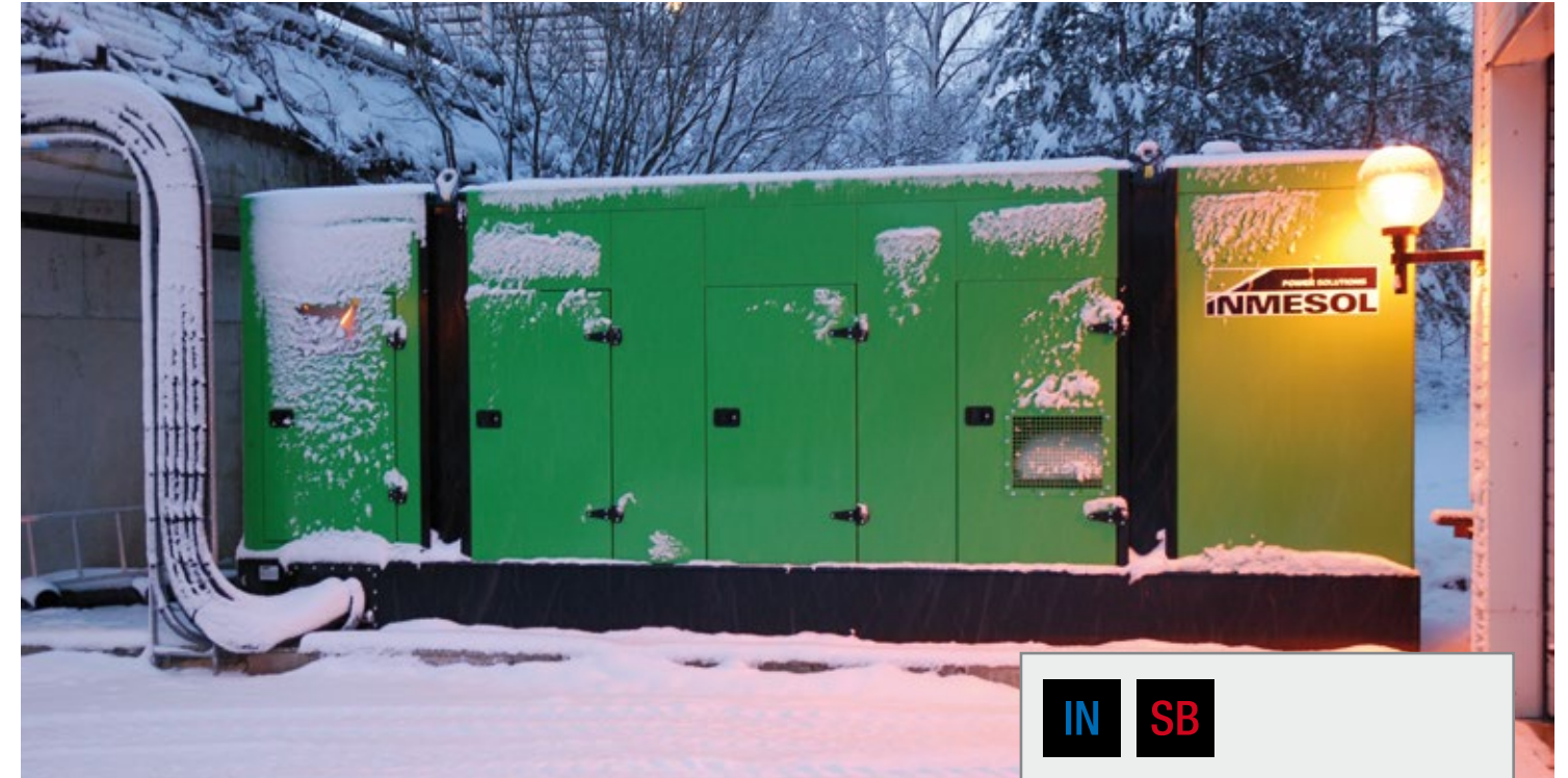
Stand-by generator set in a medicine distribution center in Sweden.
