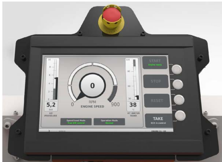
Fig 14-2 Local operator panel
